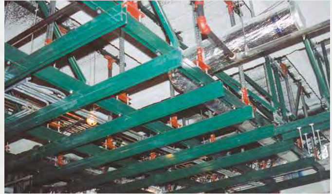
Multi-rail support system with Telespar drops.
