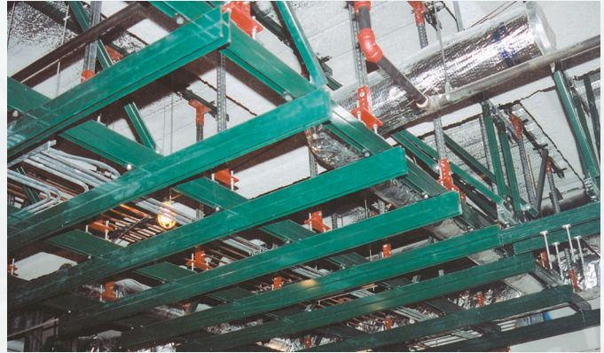
Multi-rail support system with Telespar drops.
